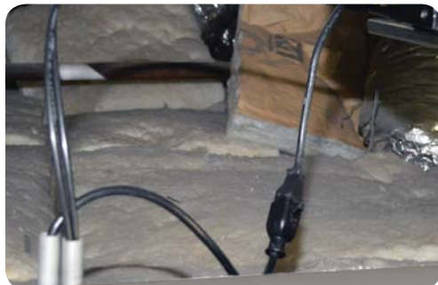
COOLER WATER AND ELECTRIC LINES IN CONDUIT
